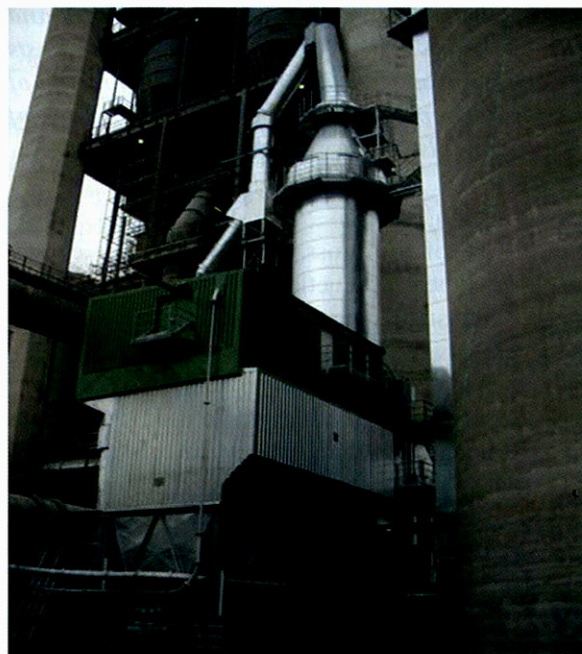
Fig 1. Holcim Lägerdorf – Eco filtering installation with evaporation cooler
