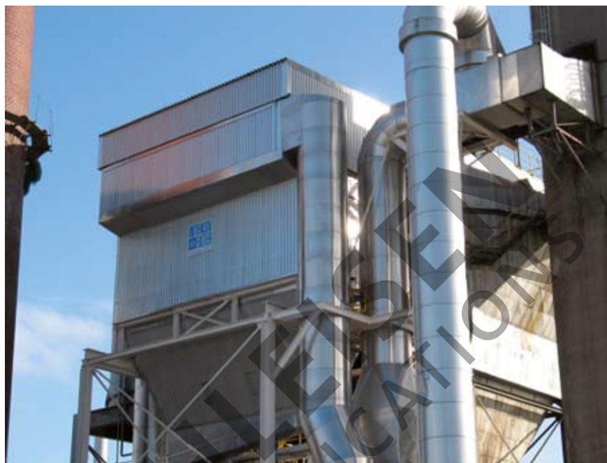
Figure 1. Waste gas treatment plant
