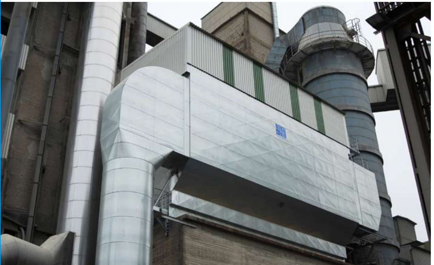
The EcoJet- bag filter in operation.
