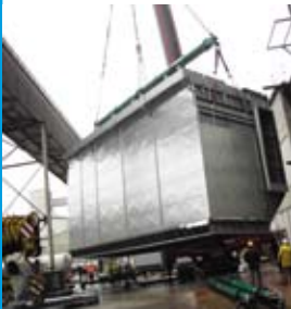
Positioning of the bag filter on the overhauled dust hopper.
