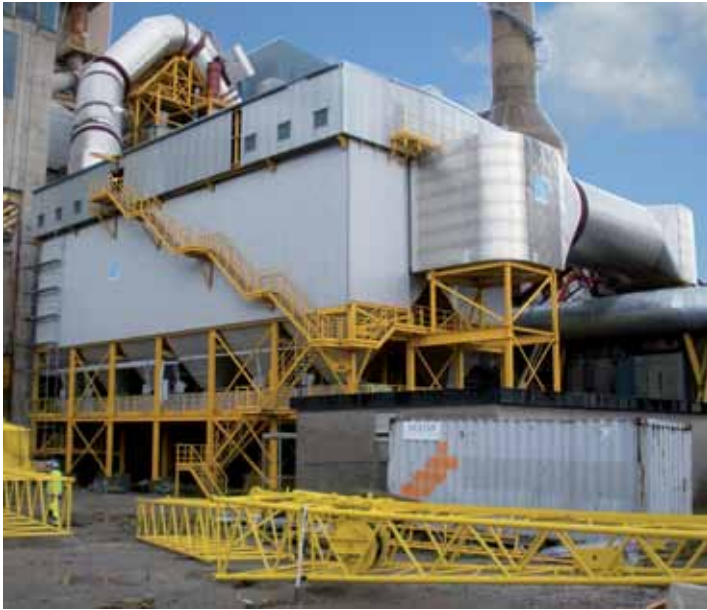
Cemeta AB, Slite plant, Sweden (Heidelberg Cement) Turnkey project ProJet mega® with offline cleaning Dust removal in a rotary kiln
