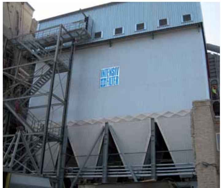
Doncement, Ukraine (Heidelberg Cement) Electrostatic filter conversion ProJet mega® with offline cleaning Dust removal in a rotary kiln
