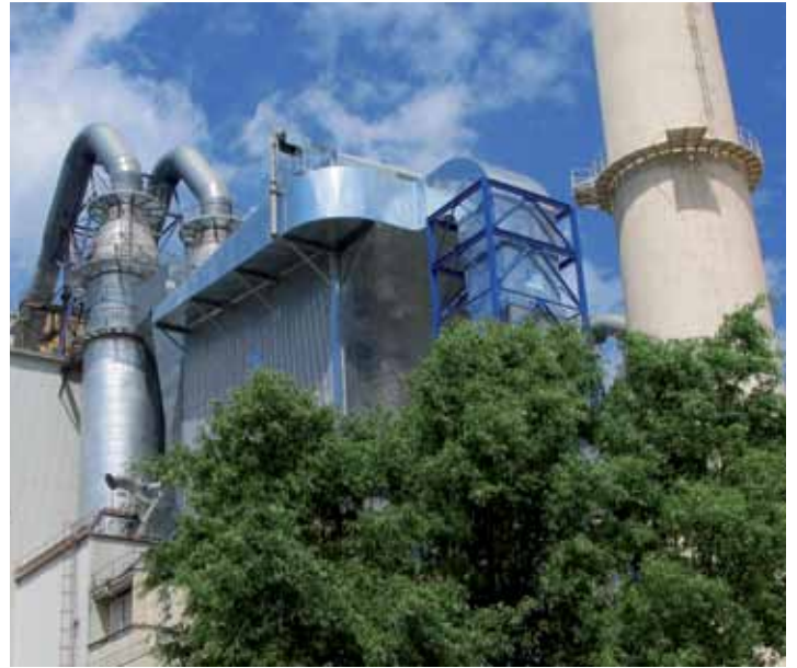
Deuna Zement GmbH, Germany (Heidelberg Cement) Electrostatic filter conversion CombiJet double row filter with semi-offline cleaning, dust removal in a rotary kiln/raw meal mill
