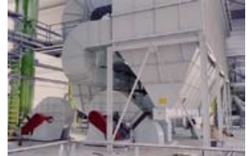
Dust removal of a fluid bed drying installation in the sugar industry
