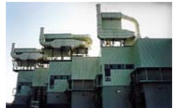
Dust removal of a waste incineration plant
