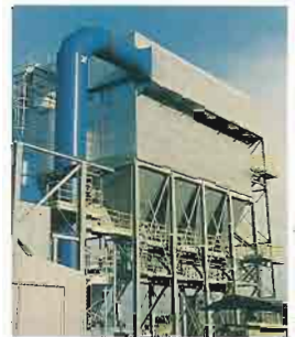
Sorption installation after a non-ferrous metal melting furnace for separation of polychlorinated hydrocarbons.
