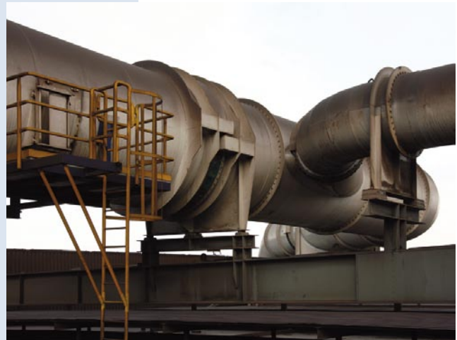
Figure 2. Junction of the crude gas collection pipe
