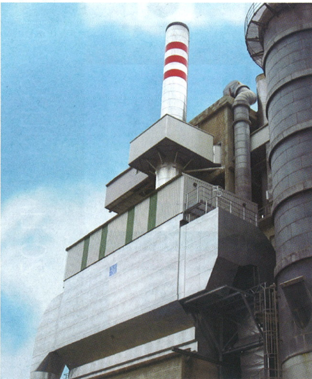
Figure 6. The installation today.
